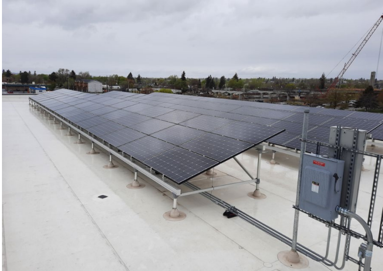
Figure 5: Solar arrays installed on the roof of building 1 during the South Wing Renovation.
